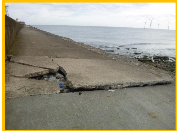
Damage to deckslab along eastern face (/C0506C01)
