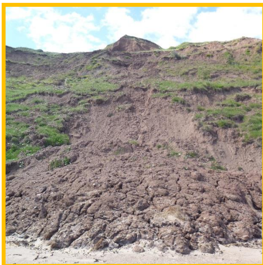
Characteristic mudslide along the toe of E55/1 .
