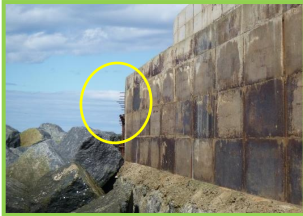
Seaward face of repair. Note exposed reinforcement. (Asset Ref No. 1221D901D0201C02)
