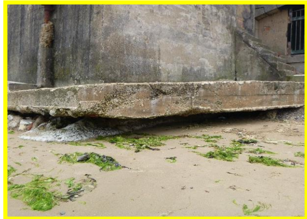
Undercut toe of Cinema seawall (/C0602C05)
