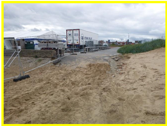
Undercutting of western corner of the asset (/C0601C01)
