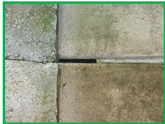
Loose and missing flexible joint sealant (/C0506C01)
