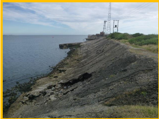
Large void in western face (/C0506C01)
