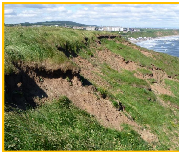
E53/2 slumping in the till layer of the cliff northeast of Saltburn (Partly Active)
