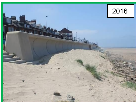
Accretion of sand and formation of embryo dunes at south eastern extent of defence in 2016 (/C0602C01)
