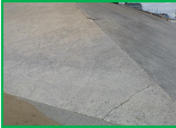
Cracking of precast slabs around access ramps (/C0602C01)
