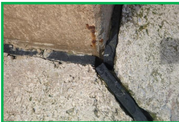
Missing flexible joint sealant in vertical joint. No sealant in horizontal joint – black filler board visible (/C0602C03)
