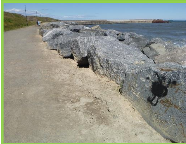
Evidence of washout of surfaced path. (Asset Ref No. 1221D901D0202C01)
