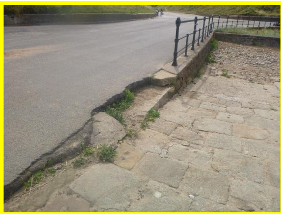
Missing coping stone exposing fill beneath promenade surface (/C0703C02)
