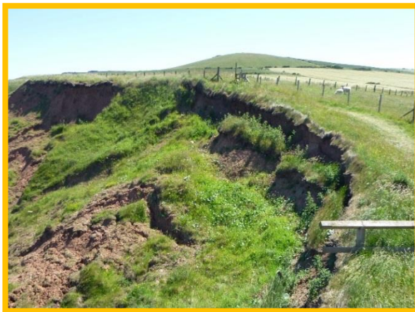
E57/7 Slumping cliffs (Partly Active)
