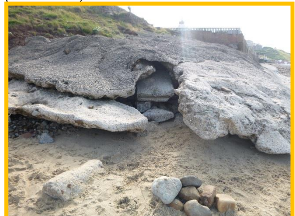
Undercutting/voiding in in situ concrete apron (/C0704C05)
