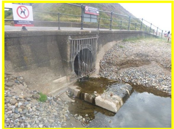
Security grille damaged (/C0703C02)
