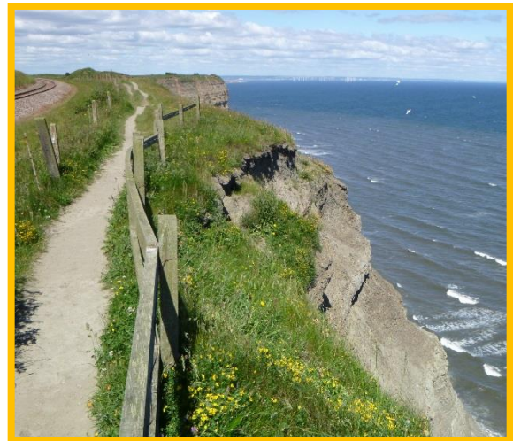
E54/3a proximity of footpath and railway line to actively eroding cliff top (Partly Active)
