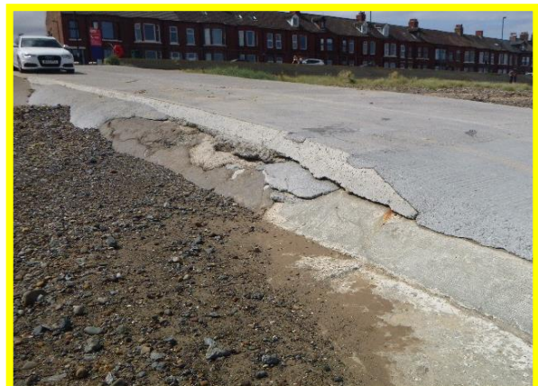
South eastern access ramp. Loss of concrete render exposing grouted stone fill beneath concrete deck slab (/C0602C01)
