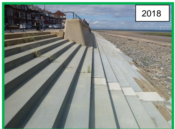
Loss of sand build up in 2018 (/C0602C01)
