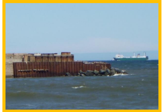
Heavily corroded sheet piles and rock armour around nose of original jetty structure.
