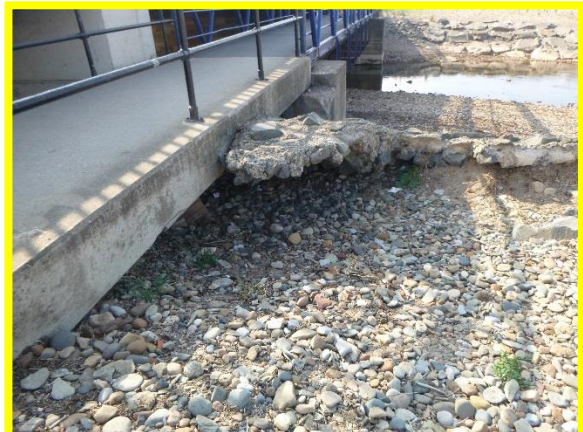
Undercutting of rock revetment apron (C0704C06)
