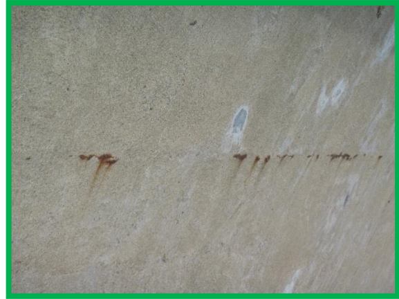
Corrosion staining in precast slabs sections around access ramps (/C0602C01)
