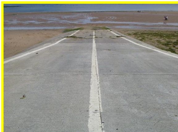
Cracking and local damage to surface of RNLI slipway (/C0602C02)
