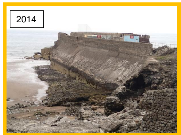
Voiding and collapse of west side of jetty structure in 2014 (Asset Ref No. 1221D901D0201C02)
