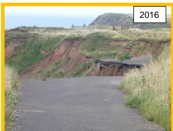
E59/3 and E59/4 Loss of road due to ongoing erosion at Cowbar Lane
