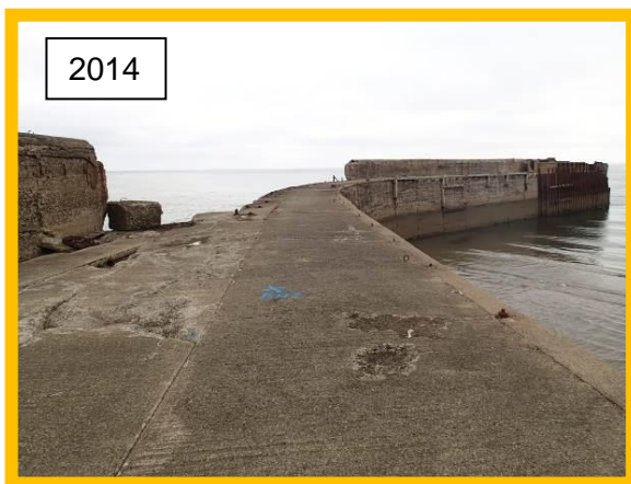
View of crest from access gate showing missing section of crest wall and damaged deck in 2014 (Asset Ref No. 1221D901D0201C02)
