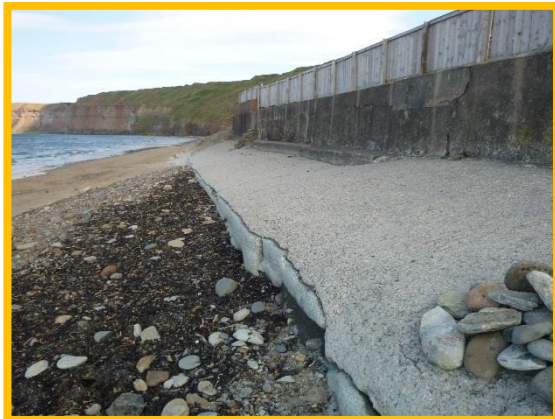
Low beach levels exposing undercutting of toe (/C0704C05)
