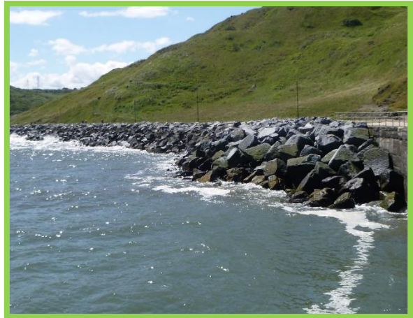
Modified rock revetment protecting inner face of jetty (Asset Ref No. 1221D901D0202C01)
