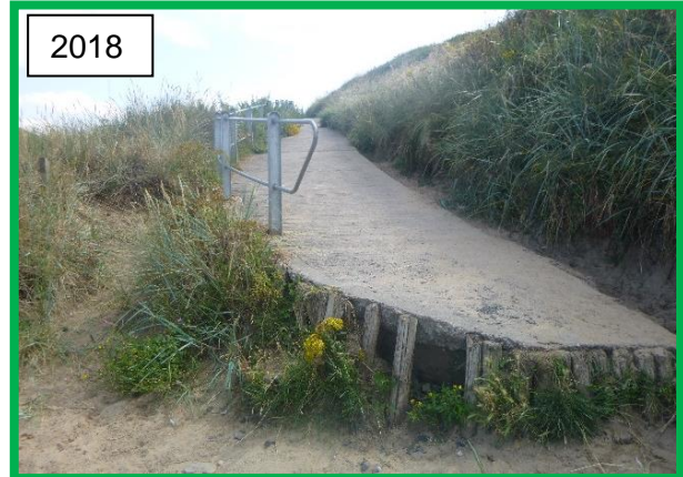
Further exposure of timber piles at foot of concrete footpath (CBU E52/6)
