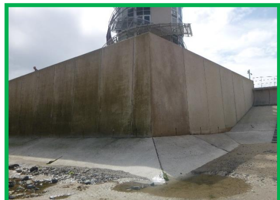
Exposed concrete apron – no sealant in joints – black filler board visible (/C0602C03)
