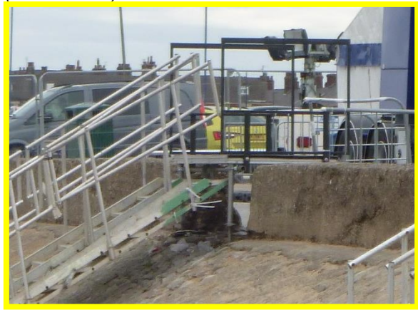
Gap in concrete wall partially visible despite being obscured by fair (/C0601C01)
